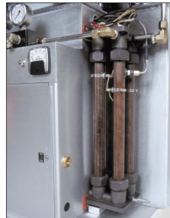
Vertically Set 6000 Watt Pre-heaters
